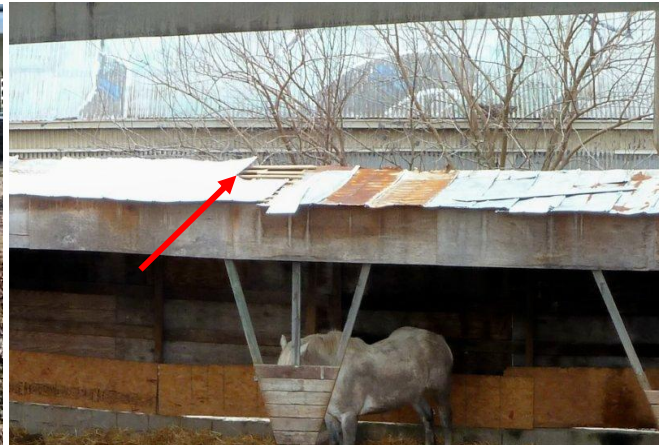
Roof in disrepair
