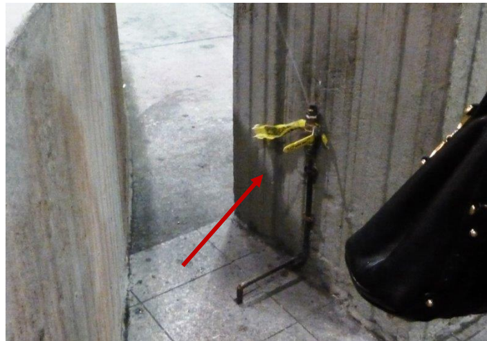
Former water source disabled
